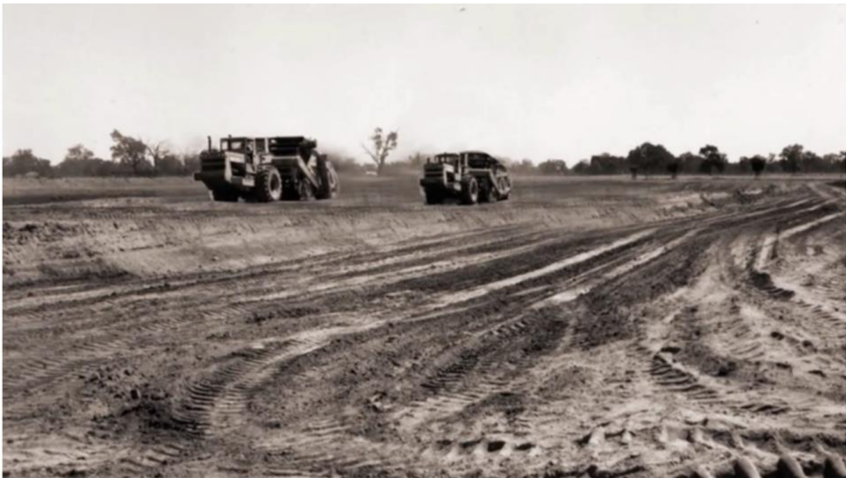
Figure 11. The construction of Lake Mokoan, 1967-1971, showing significant ground disturbance Source: Winton Wetlands, https://wintonwetlands.org.au/learn/european-history/ .
